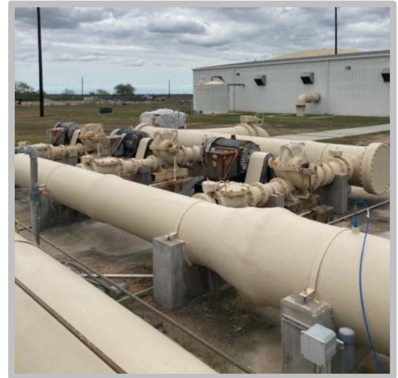
MF Transfer Pump Station
