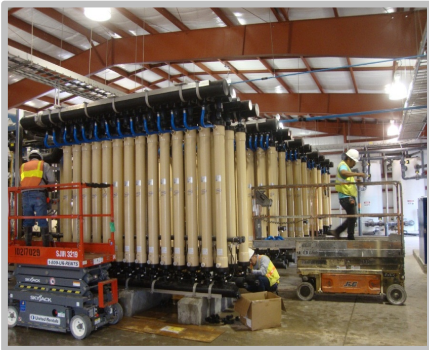
Pretreatment and RO expansion
